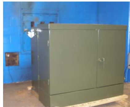
Figure 1 - Pad Mounted Transformer
